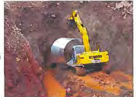
Figure #3: Installation of large diameter culvert at Level F following portal excavation.
