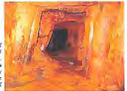
Figure #4: View looking up Level F access. Photo shows timber supports and significant iron hydroxide build up.
